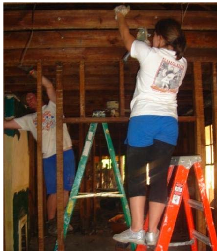
United Methodist college volunteers from Georgia prepare this Katrina-damaged home in New Orleans to be renovated. Credit: DNN/Jim Skillington
