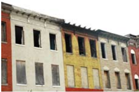
These burned-out vacant homes stand just a block from the new ones at Preston Place. They too have been acquired by BUILD and are slated for demolition. (Photo Andy Cook)
